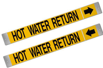
PIPE MARKERS PLACED ON HOT WATER PIPES
